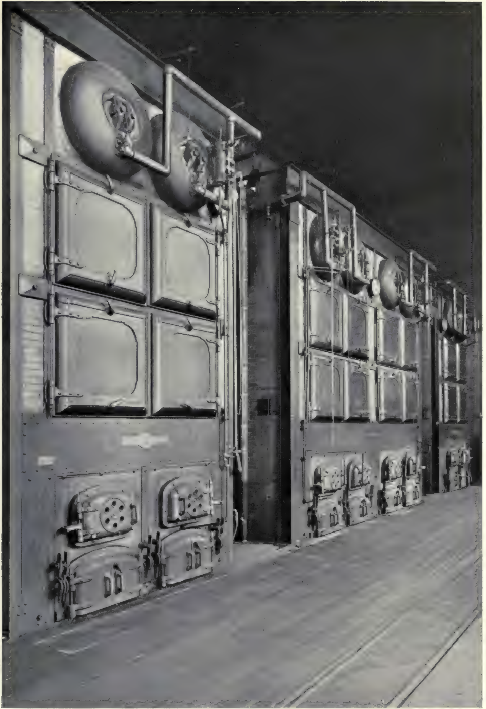
SOUTH PITTSBURGH, PA., WATER CO. BABCOCK & WILCOX SUPERHEATERS INSTALLED IN 1200 HORSE POWER OF BABCOCK & WILCOX BOILERS
